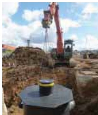
Due to its light weight and robust build, the SDS Aqua-Swirl™ hydrodynamic separator could be lifted and maneuvered easily into position using the excavation equipment already on site. Photo by SDS Ltd.
